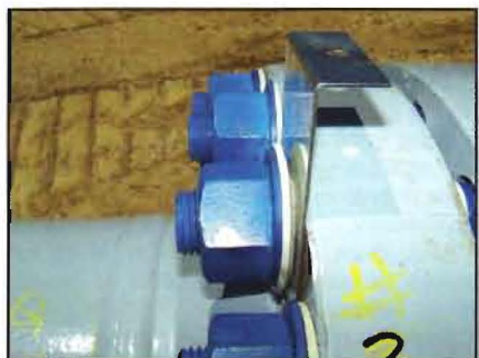
Figure 5.: Over-compressed white isolation washer.
